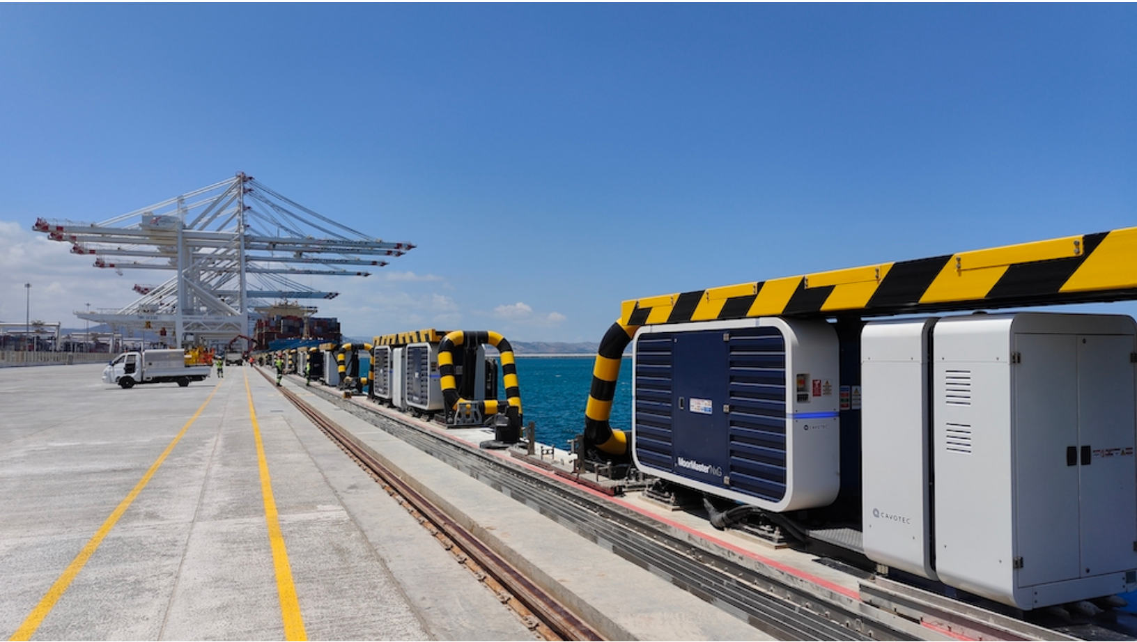
Cavotec MoorMaster NxG units at AMP Terminals MedPort Tangier
