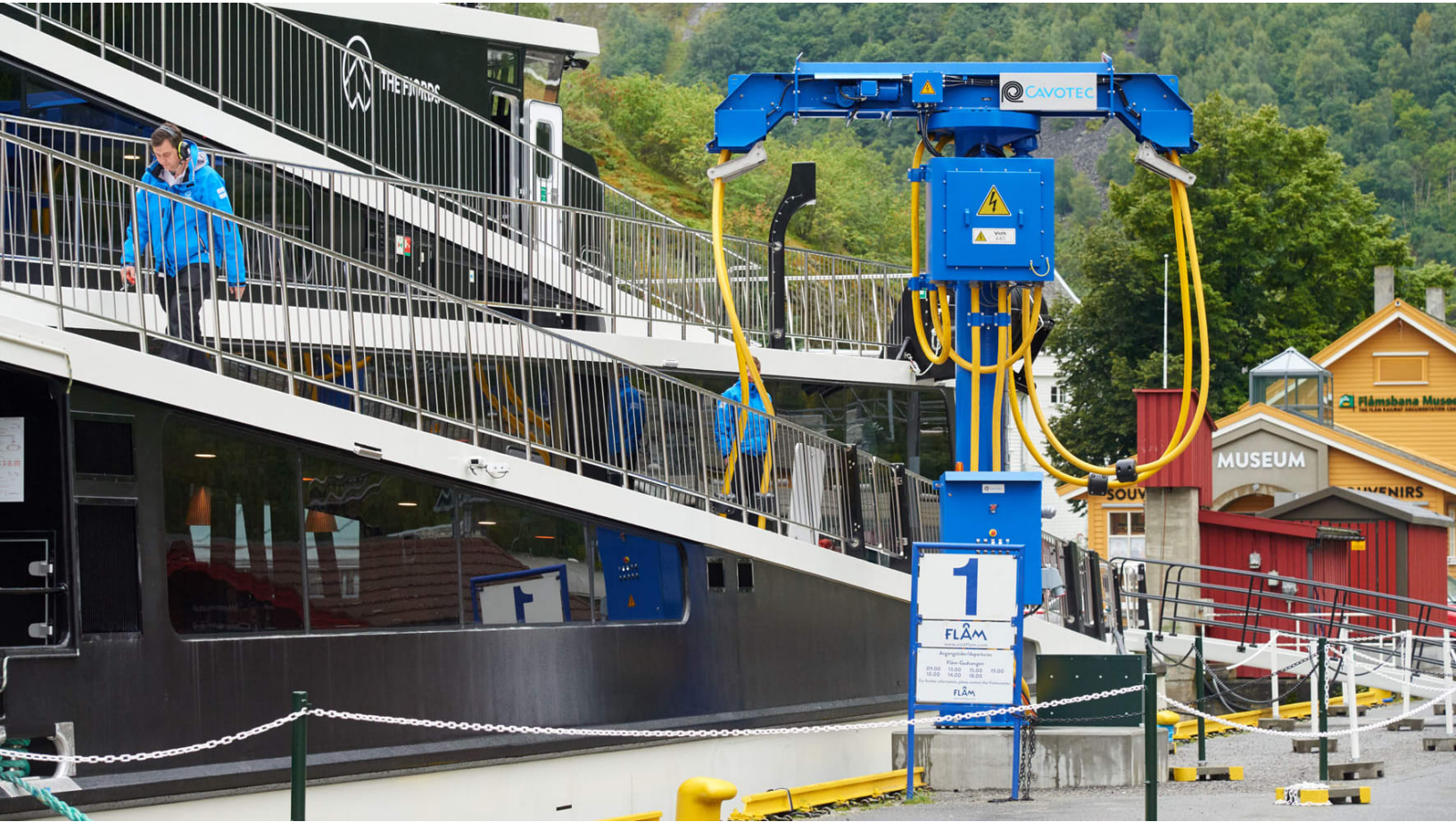
All set: a shore power dispenser unit charging the Vision of the Fjords at the Flåm berth in Norway.
