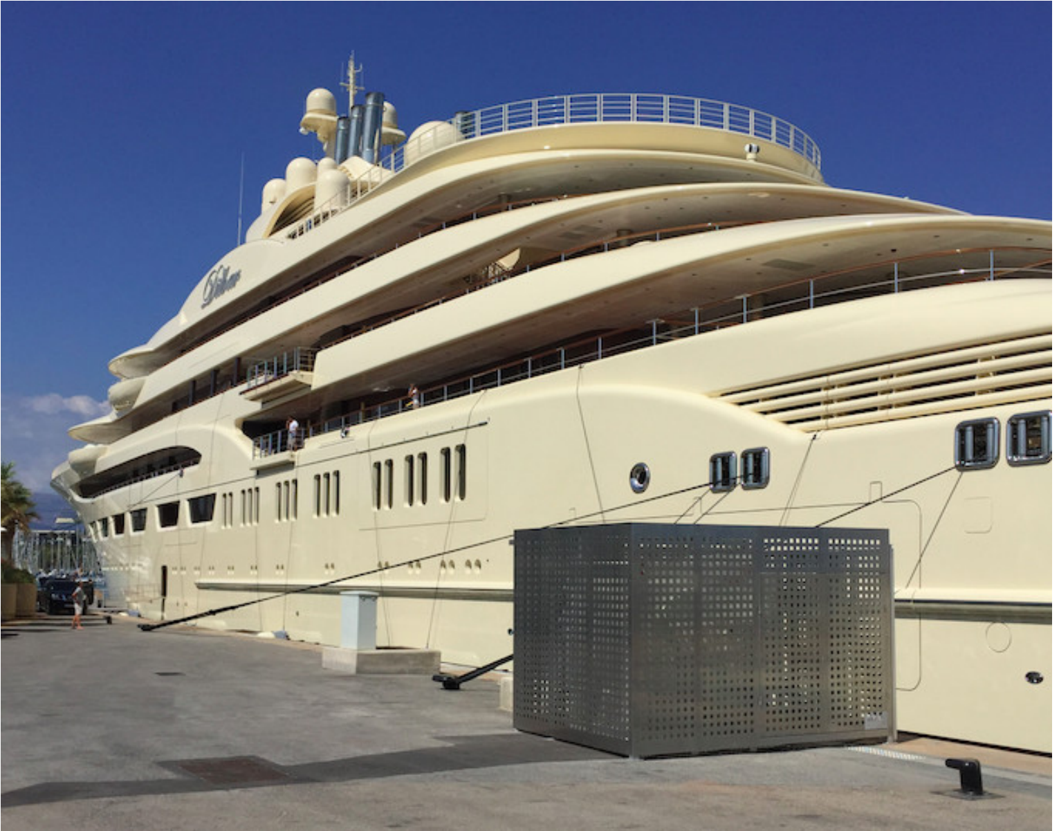
Living the life: the enclosed AMP unit and the Dilbar at Vauban.
