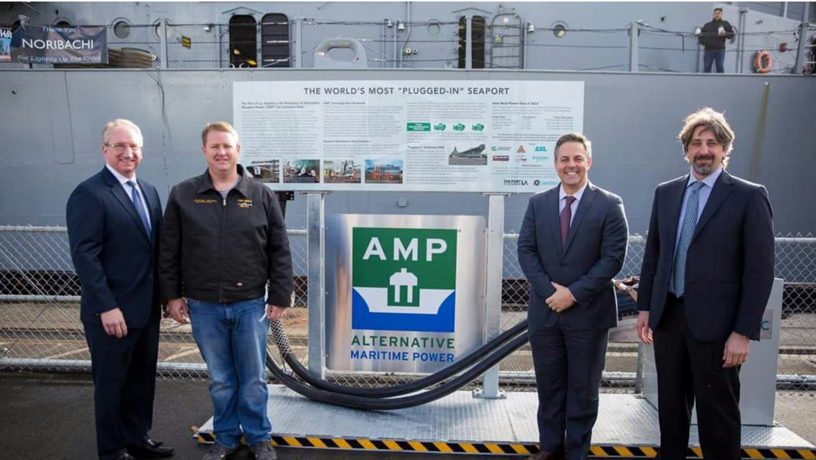
From left to right: Port of LA Executive Director, Gene Seroka; Jonathan Williams President & CEO Battleship Iowa; LA City Councilman Joe Buscaino; and Cavotec's Luciano Corbetta. Photo used by kind permission of POLA.
